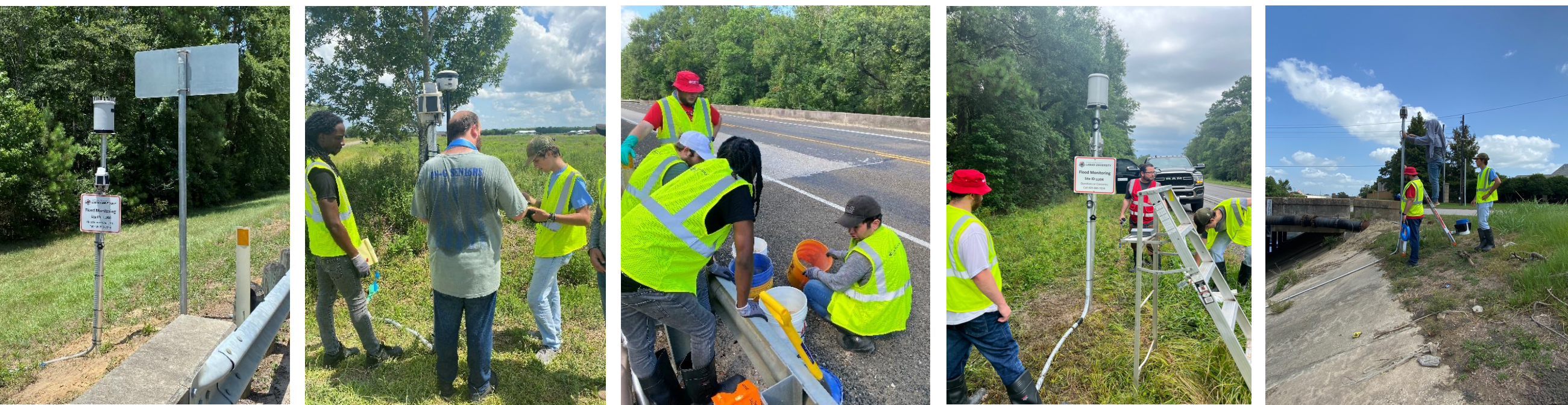
Fig 4: Flood monitoring sites installation, field surveying and maintenance.
