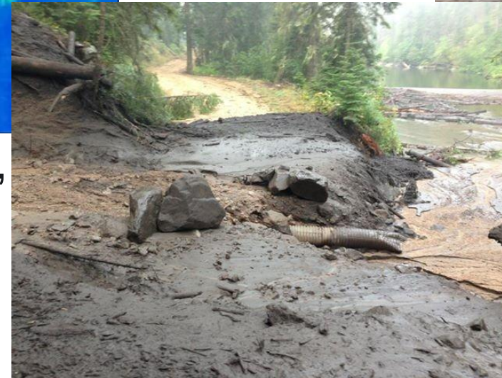
Extreme Weather- related Water Hazards
