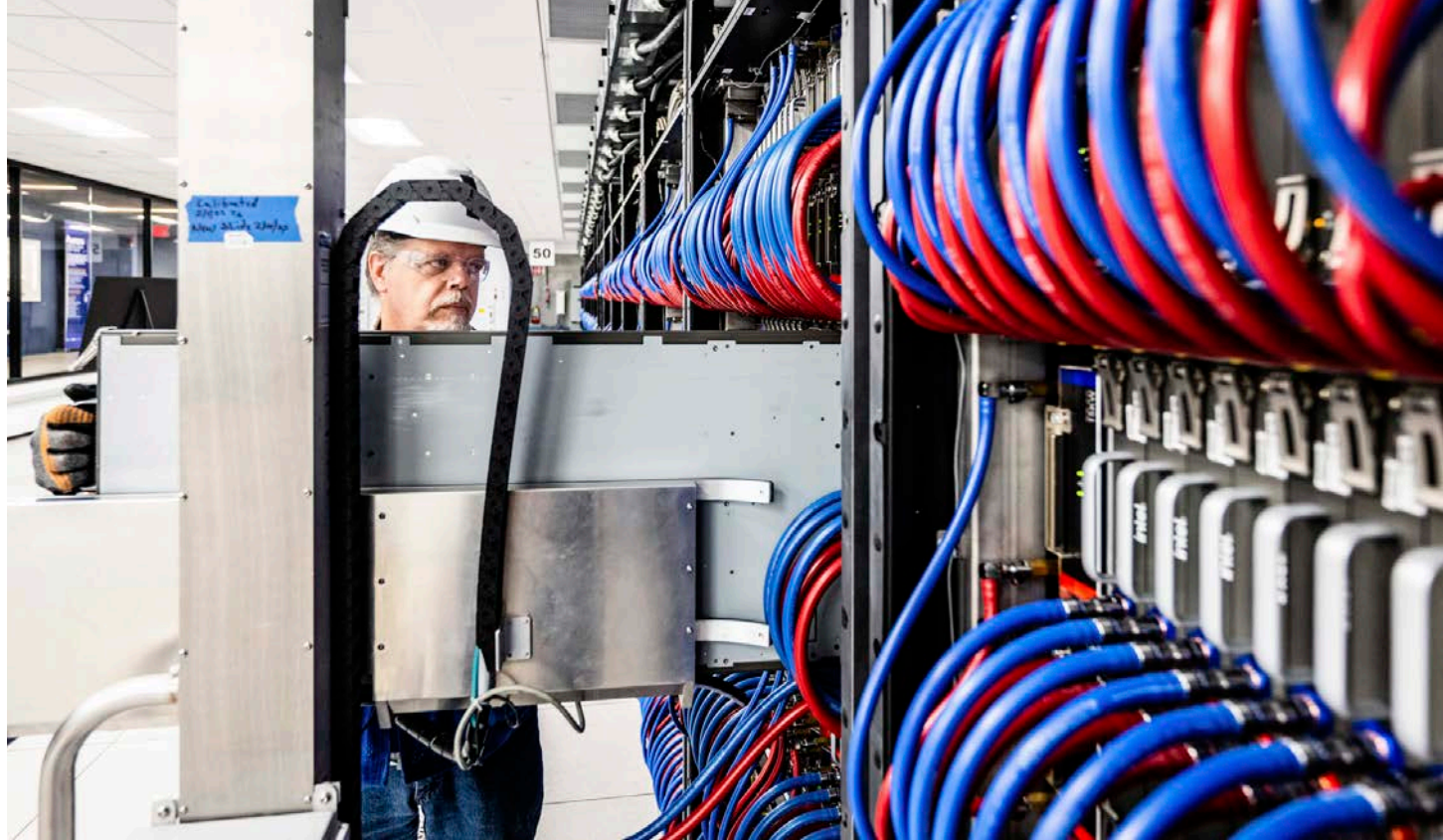
Aurora supercomputer at Argonne National Laboratory. [Courtesy Argonne National Laboratory]
