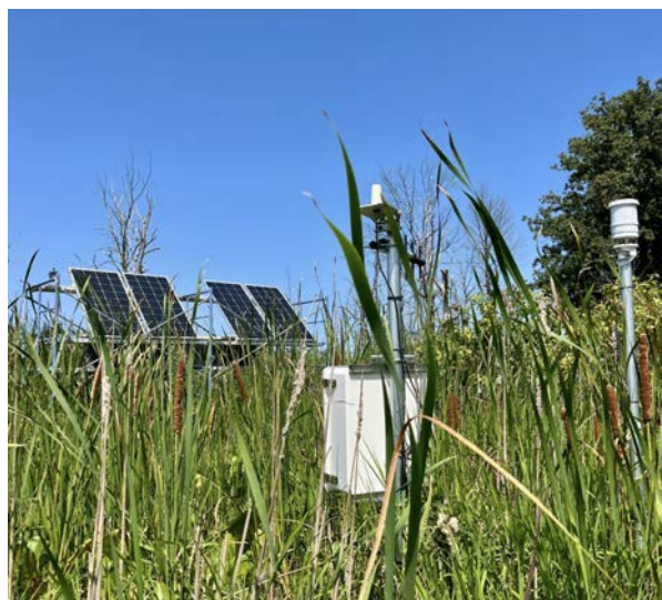
Fig. 2.3. Gathering Continuous Ecological Data Demands Energy Infrastructure and Data Logging. Solar panels (left) supply power to sensors and dataloggers at one of the COMPASS-FME wetland research sites in Ohio. The pole (right) includes sensors for photosynthetically active radiation, temperature, relative humidity, wind, and precipitation. The datalogger in the white box (center) collects these data as well as data from unseen belowground and aboveground sensors such as tree sap, soil moisture, temperature, and other environmental conditions. [Courtesy Nick Ward, Pacific Northwest National Laboratory]
